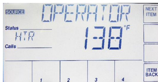
Figure 10-8 Setting the Setpoint
