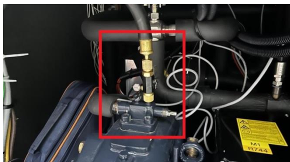
Vacuum pump hose connection
