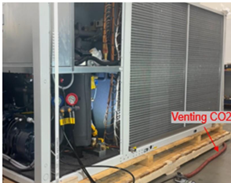
REFRIGERATION MANIFOLD w/ DISCHARGE HOSE ATTACHED TO THE CENTER VALVE
