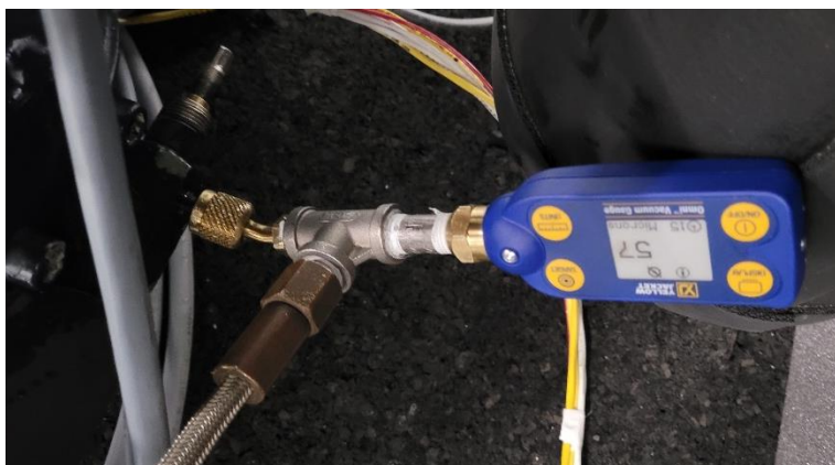
Micron Gauge attachment to discharge compressor
