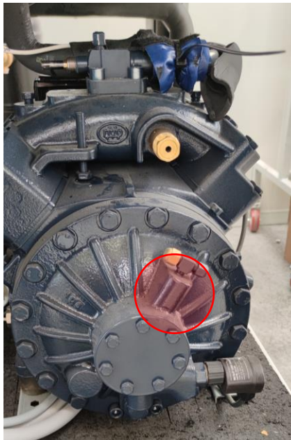
Compressor Oil Pump Connection
