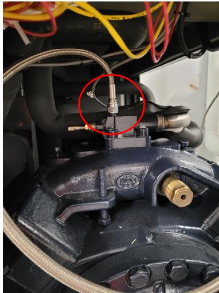
Compressor Discharge Valve
